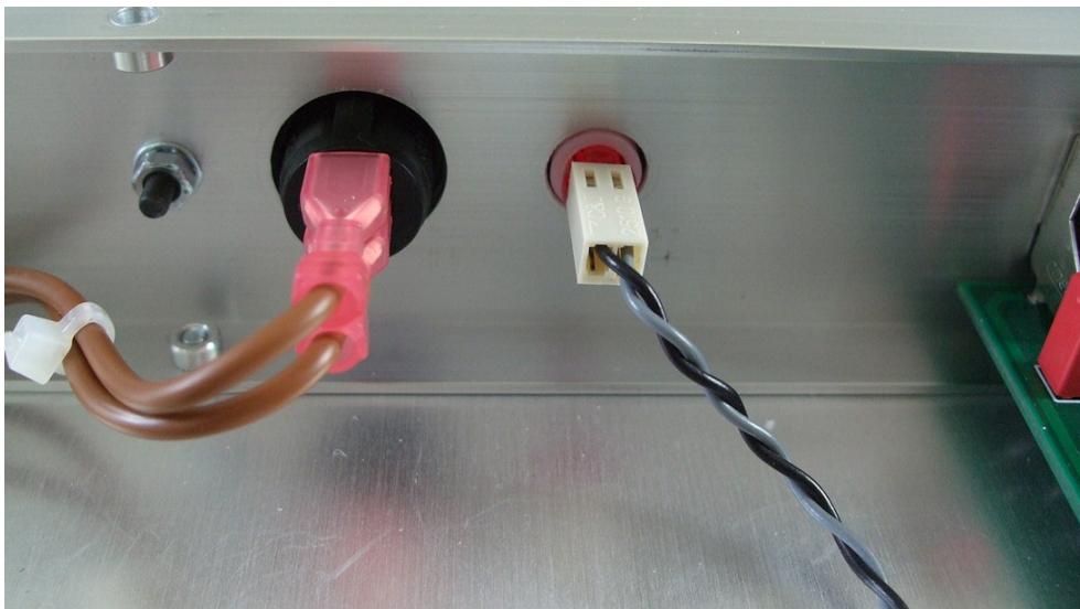
The power on LED fitted into a LED clip. The twisted pair of wires connect back to the RPSU but could go back to the PWR location on the main board.
